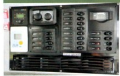
The EarthCruiser control centre
